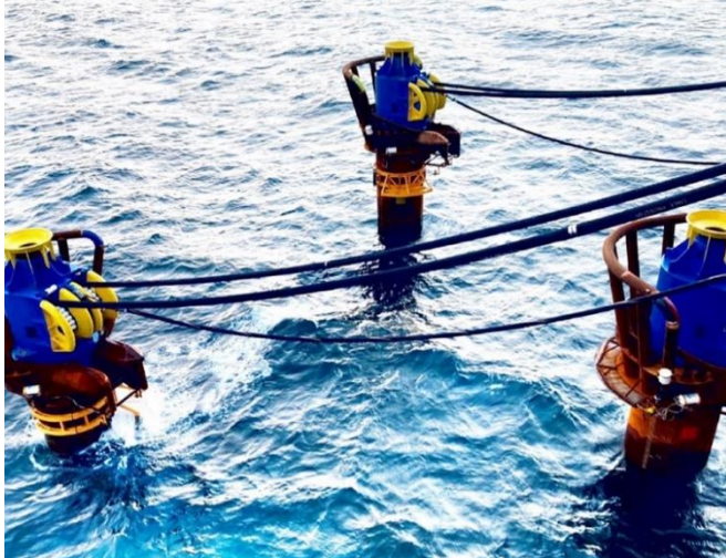
(2) With up to three drilling rigs operating simultaneously, piles are anchored safely and efficiently in challenging soil conditions. © BAUER Group
