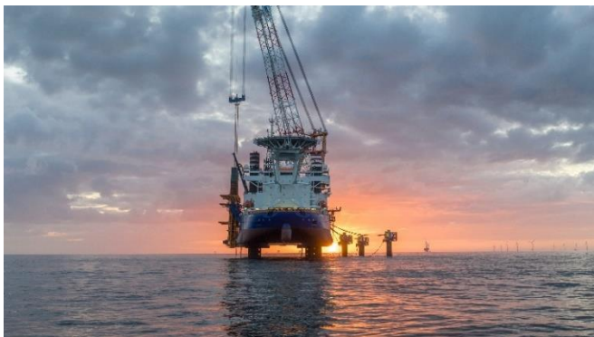
(3) Passing the reinforcement test: Bauer drilled a total of 190 piles off the coast of France using the Dive Drill method. © Van Oord
